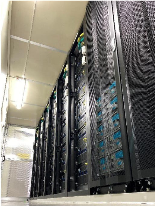
Photographs inside the data center
